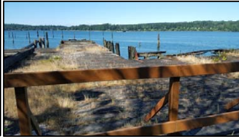
Former Log Transfer Facility, the first structure to be demolished this year
